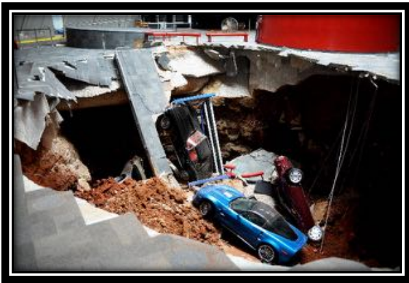
Large sink hole at the museum Feb. 12, 2014
